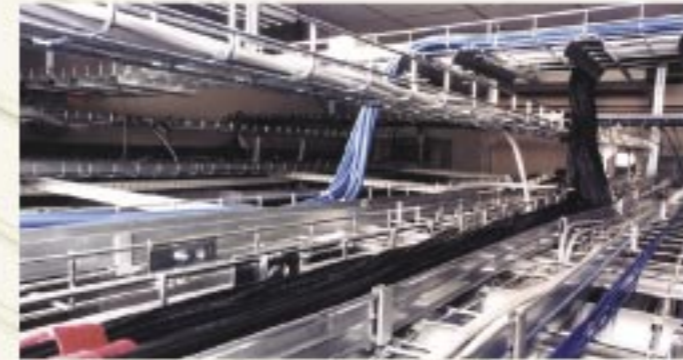
IT cable channelling - data centres Cables moved, added and changed. In safe lanes with the Defem "Tore Concept".
