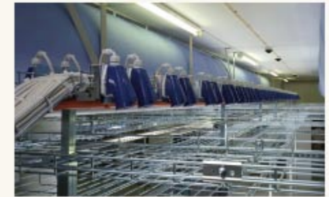
Telecom Transmission room I Separate levels for separate cables Full cable control with the "Tore Concept".
