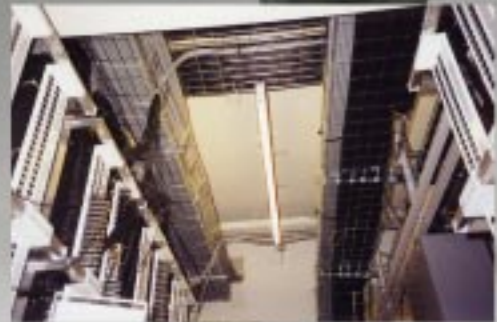
Extreme cable loads - possible with Defem
