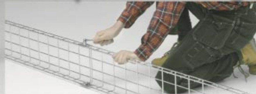
Most joinings are made at floor level. One man lifts 3 joined sections = 7,5 metre. Two men lift 5 joined sections = 12,5 metre
