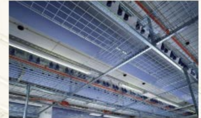
Telecom Transmission room II The safest method for future flexibility: The Tore concept ( www.defem.com/applications ).
