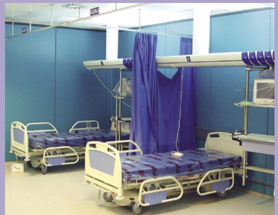
Basurto Hospital - Recovery unit - Bilbao (E)
