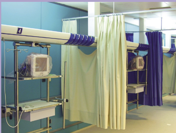
Basurto Hospital - Recovery unit - Bilbao (E)
